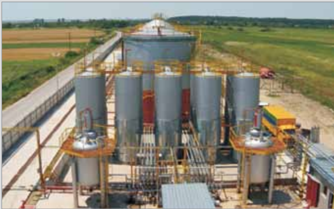
WASTE OIL REFINING
